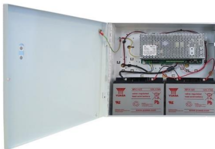
Figure 7 – Battery backup supply
